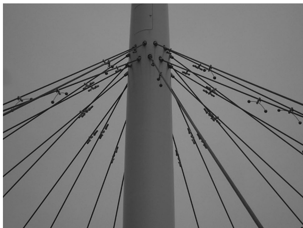
Fig. 13 Stockbridge-type dampers installed on the stay cables of the Hovenring Bridge [110]
