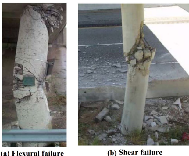
Fig. 10 Typical failures occurred in bridge columns at the mid-height under vehicle collisions [78]
