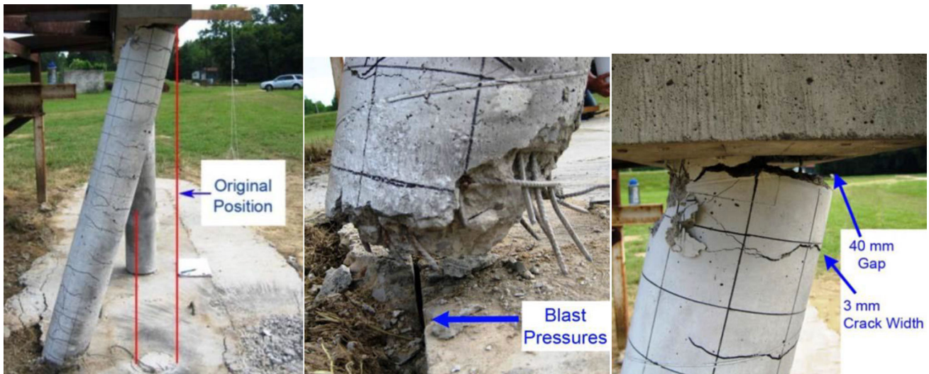
Fig. 10 Shear failure at the base and top of the RC column [72]
