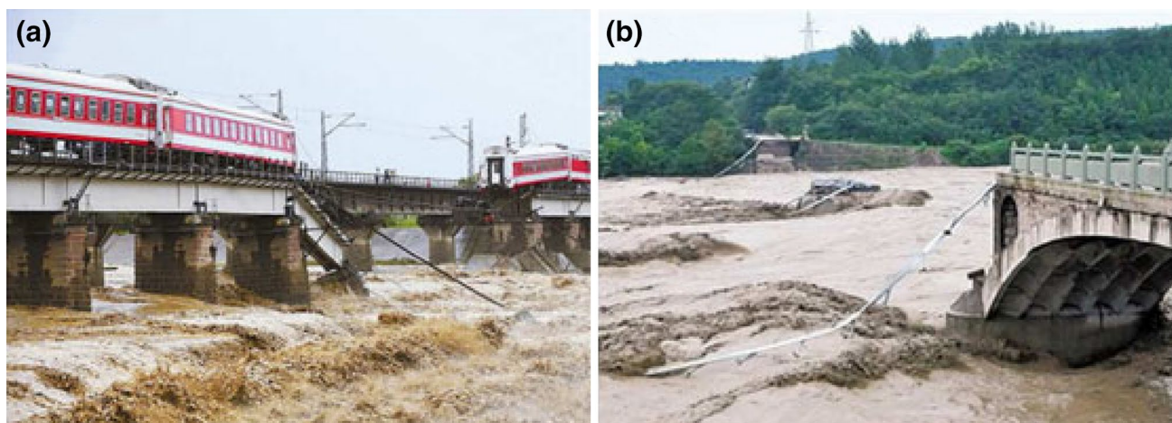
Fig. 1 Scour-induced bridge collapses a Shi-Ting-Jiang Bridge and b Pan-Jiang Bridge
