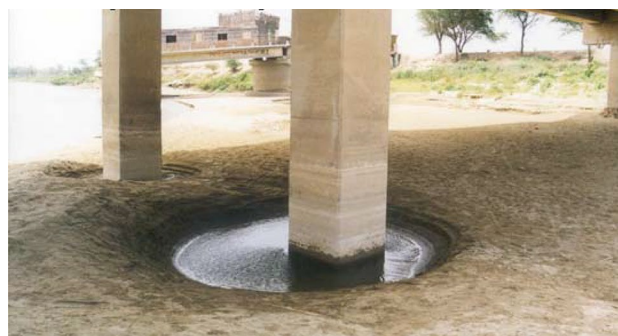
Fig. 2 Photograph of local scour at rectangular piers
