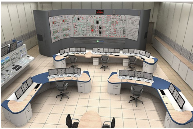
Fig. 19 Digitalized main control room of the APR1400 [125]
