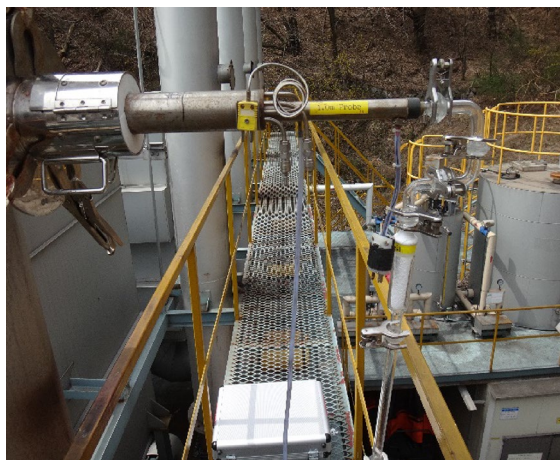
Fig. 2 Current Status of Cremation Facility Sampling Site Equipment Installation
