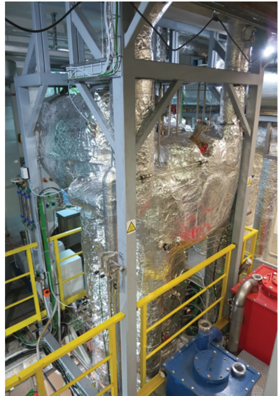
Fig. 5. Photograph of the upper part of the advanced pilot facility at TU Wien.
