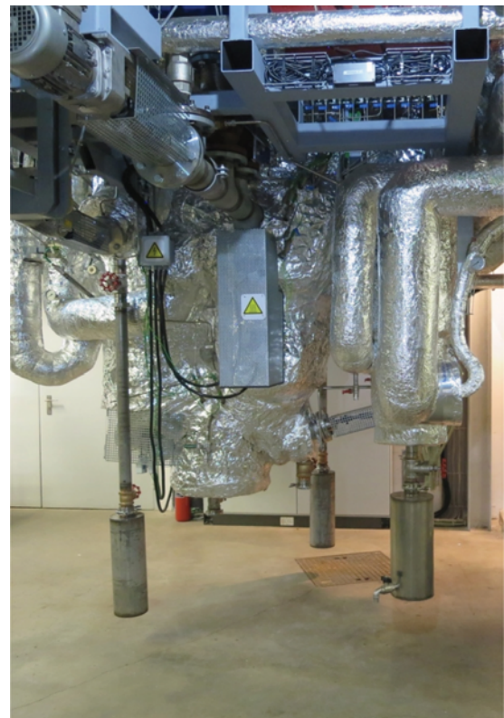
Fig. 6. Photograph of the lower part of the advanced pilot facility at TU Wien.
