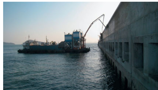
Fig. 1 Perforated wall breakwater of the Dalian Chemical Production Terminal, China, in Huang et al. (2011)
