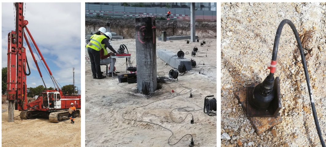
Fig. 11 Experimental test site: (a) pile driving rig Junttan PMx25 equipped with the hydraulic impact hammer SHK110-7; (b) and (c) unidirectional accelerometers placed along the ground surface
