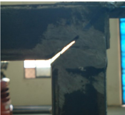
Fig. 10 Zoom view of damaged structure 20 mm crack
