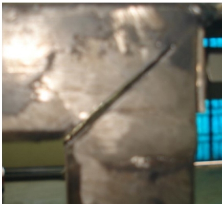
Fig. 11 Zoom view of damaged structure 30 mm crack
