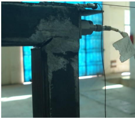
Fig. 9 Zoom view of damaged structure 10 mm crack
