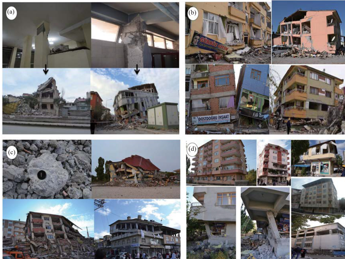
Fig. 10 Building damage caused by building irregularities after 2011 Van earthquakes (a: short column; b: soft story; c: concrete strength; d: heavy overhang)
