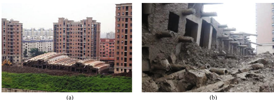
Fig. 12 Collapsed high-rise apartment building—result of improper construction
