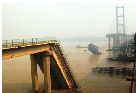
Fig. 14 Collapsed Jiujiang Bridge under ship impact (Photo by CFP)
