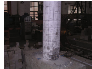
(a) Specimen A10 after loose concrete removal
