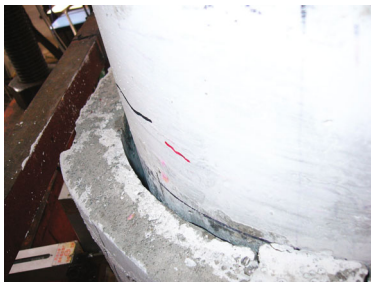
(b) Debonding failure between the concrete jacket and existing pier
