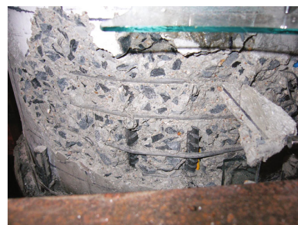
(b) Concrete spalling and longitudinal bar buckling damages
