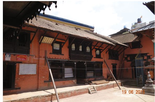
Fig. 13 Leaning outward of the wall in Hindu temple of living Buddha in Katmandu
