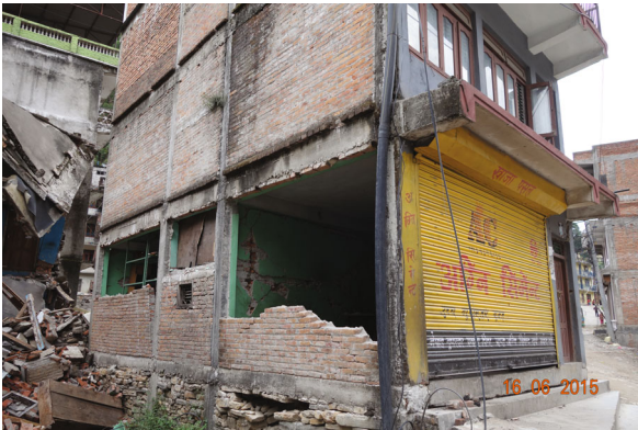
Fig. 6 Damage of the bottom infill walls of a RC frame structure
