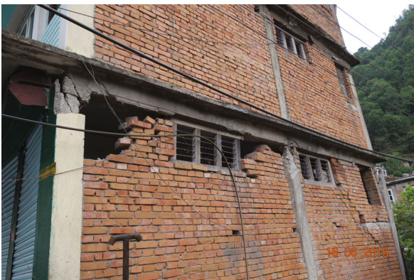
Fig. 9 Serious damage of the column capitals at the bottom of RC frame structure
