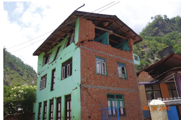
Fig. 11 Serious damage of a brick-wood structure in high intensity regions
