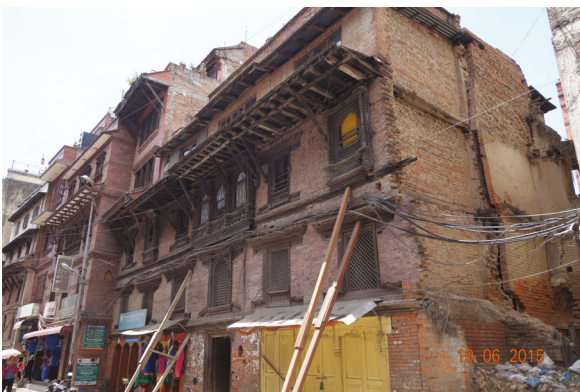
Fig. 14 Inclining outward and partial collapse of the wall in a traditional brick-wood structure in Katmandu
