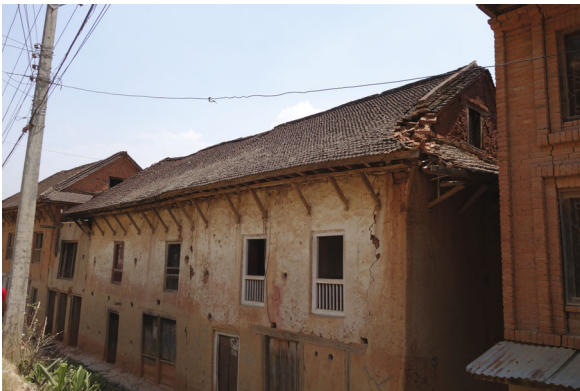
Fig. 12 Moderate damage of the brick-wood structure in Intensity VII areas
