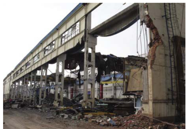
Fig. 10 Damaged factory building of Dongfang Steam Turbine Works in Hanwang Town
