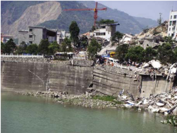
Fig. 5 Building collapse and river bank damage caused by fault dislocation in Beichuan County town
