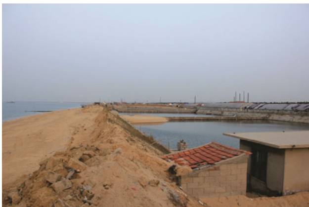
Fig.11 The picture that shows breeding pools destroyed the shoreline structures.
