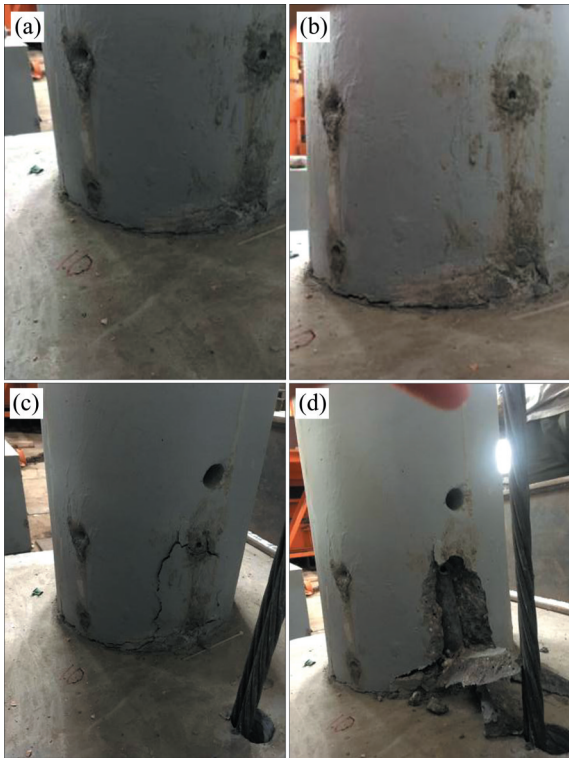
Figure 6 Damage of the GS specimen: (a) Concrete cracking at the joint of pier bottom and bearing platform; (b) Widening of concrete cracking at the joint of pier bottom and bearing platform; (c) The concrete of the outer protective layer at the position of the grouting sleeve is cracked; (d) The concrete of the outer protective layer at the position of the grouting sleeve is peeled off
