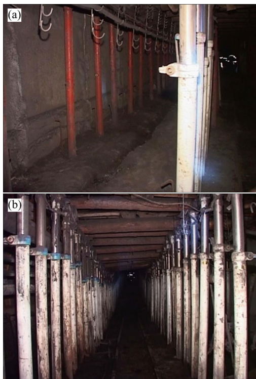
Figure 13 Images of E1403's gob-side entry retaining: (a) Filling wall; (b) Full view
