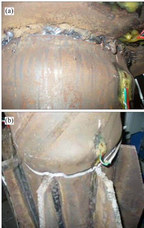
Fig. 11 CSCKJ7 structure failure diagram: (a) Column top; (b) Column heel
