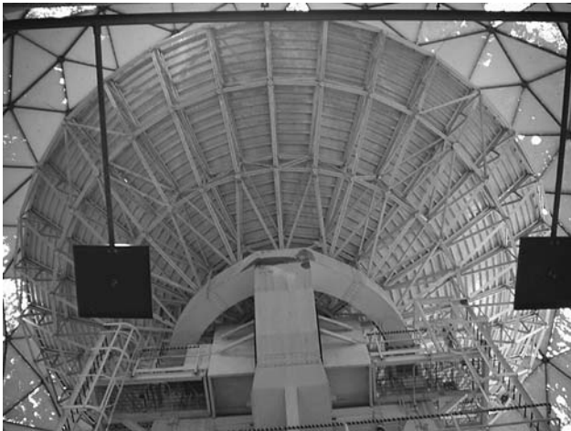
Figure 2. Inside the last-remaining Nurrungar radome. The giant 26-m telemetry dish stands dormant, protected from the harsh desert climate by its exterior Kevlar shell
