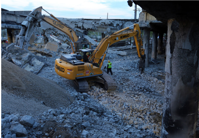
Fig. 1 Post fire damage in I-85 bridge in Atlanta, GA, USA (courtesy of GDoT).
