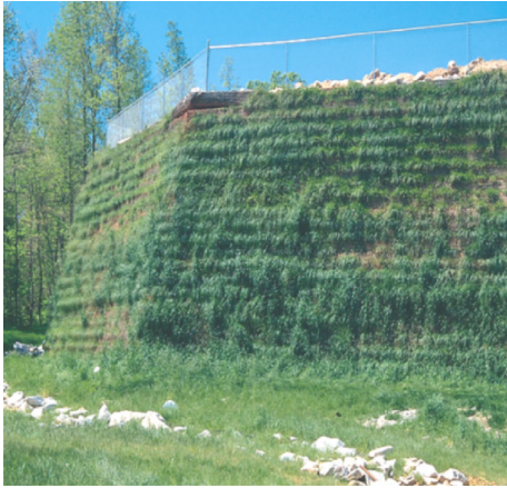
Fig. 9 Stabilized vegetated steep slope with welded-wire baskets and wrapped-around geogrid (courtesy of tensar international)
