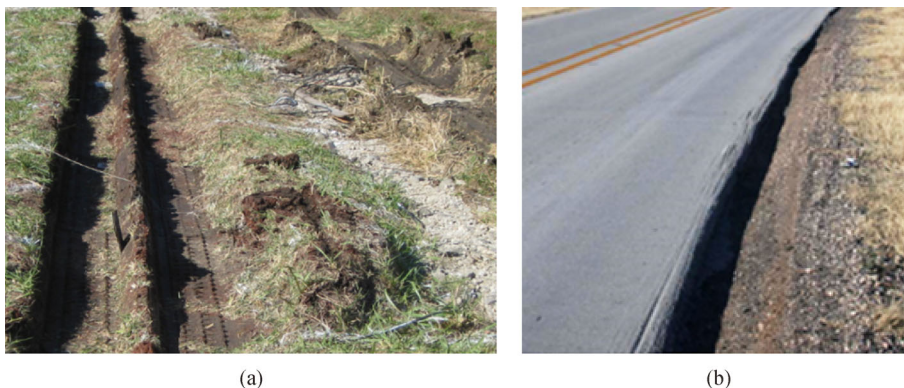
Fig. 1 Rutting and erosion of unpaved shoulders. (a) Rutting; (b) erosion
