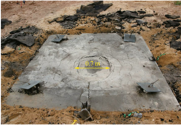
Fig. 20 Damage of proposed multi-layer pavement after blast (after removing AC layer)
