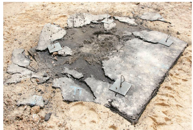
Fig. 19 Damage of the multi-layer pavement after blast load with top layer AC in place
