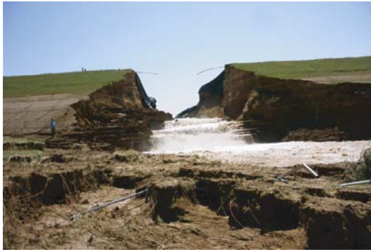
Fig. 10 Downstream view of dam after failure
