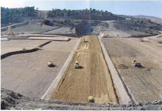
Fig. 1 Photograph of Lechago Dam showing the clay core, the filters and the rockfill shoulders
