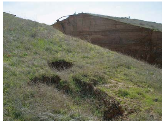
Fig. 12 Field indicators of the collapse potential of the fill
