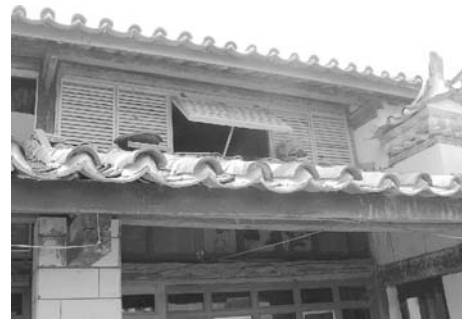
Fig. 14 Shutter for ventilation and day lighting
