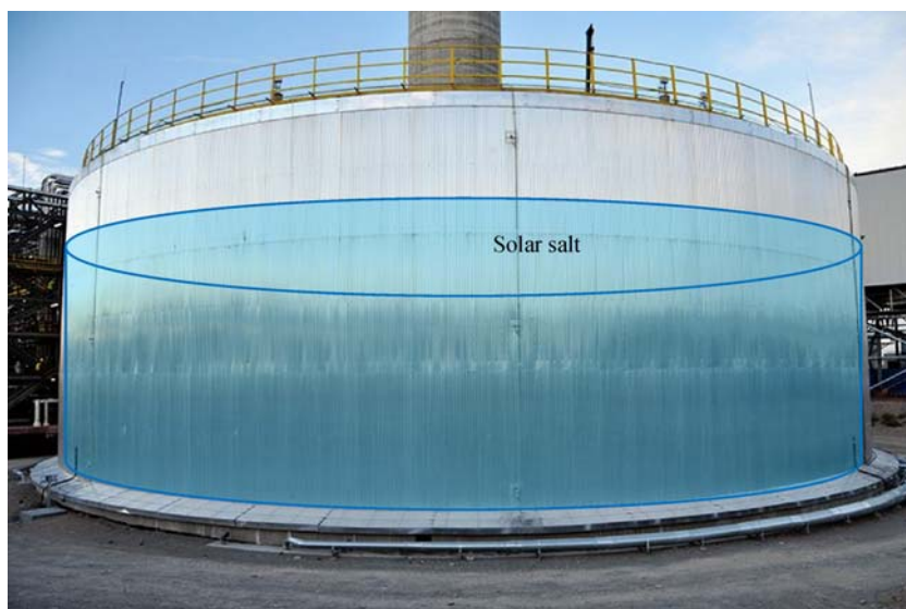
Fig. 3 A molten salt storage tank (container) for the Crescent Dunes solar power plant. Size of tank: 12.2 m tall and 42.7 m in diameter; storage capacity: 32000 tons molten salt (source: SolarReserve)
