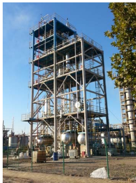
Fig. 3 Pilot plant of hydrogen peroxide production in Shijiazhuang
