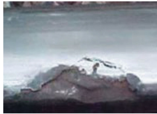
Fig. 15 Shelling/Spalling defect at rail surface [31]
