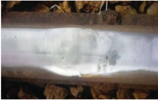
Fig. 19 Small defect consisting of wheel burns at Urban LRT
