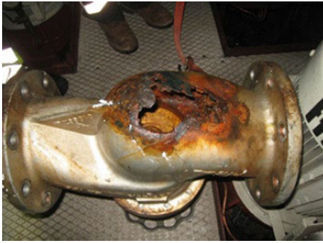
Fig. 3 Heavy corrosion on the bottom of a check valve (DNV)
