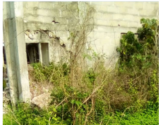
Fig. 6 Cracks drawing from the foundation of the building
