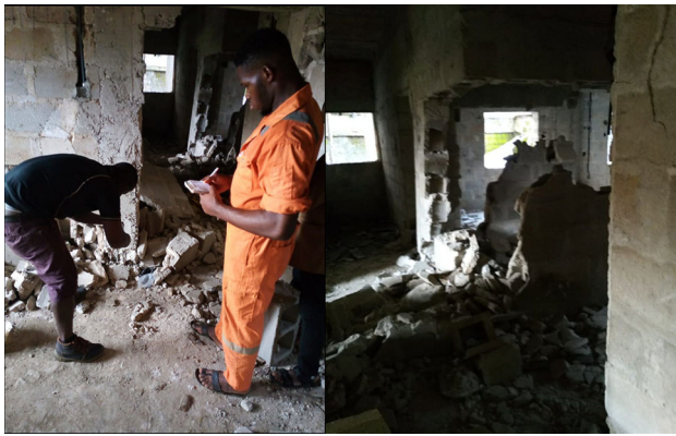
Fig. 5 Cracks at partition walls of the case study building
