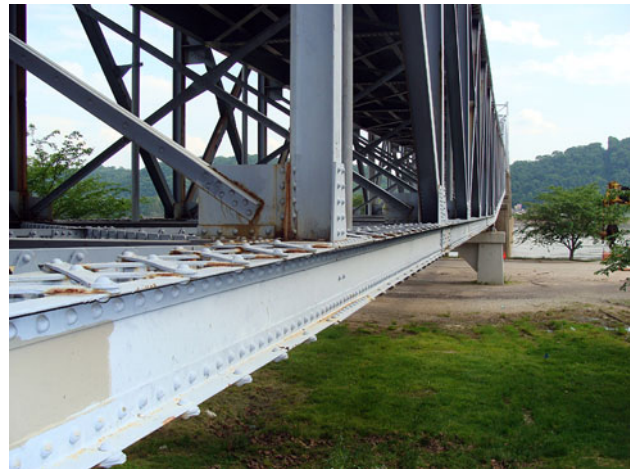
Approach span leading to the Milton-Madison Bridge in southern Indiana, which will be demolished in stages. Photo courtesy of Purdue School of Civil Engineering/Ryan Sherman
