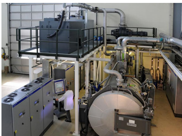
Fig. 1 New LPPS-TF facility at the Forschungszentrum Jülich
