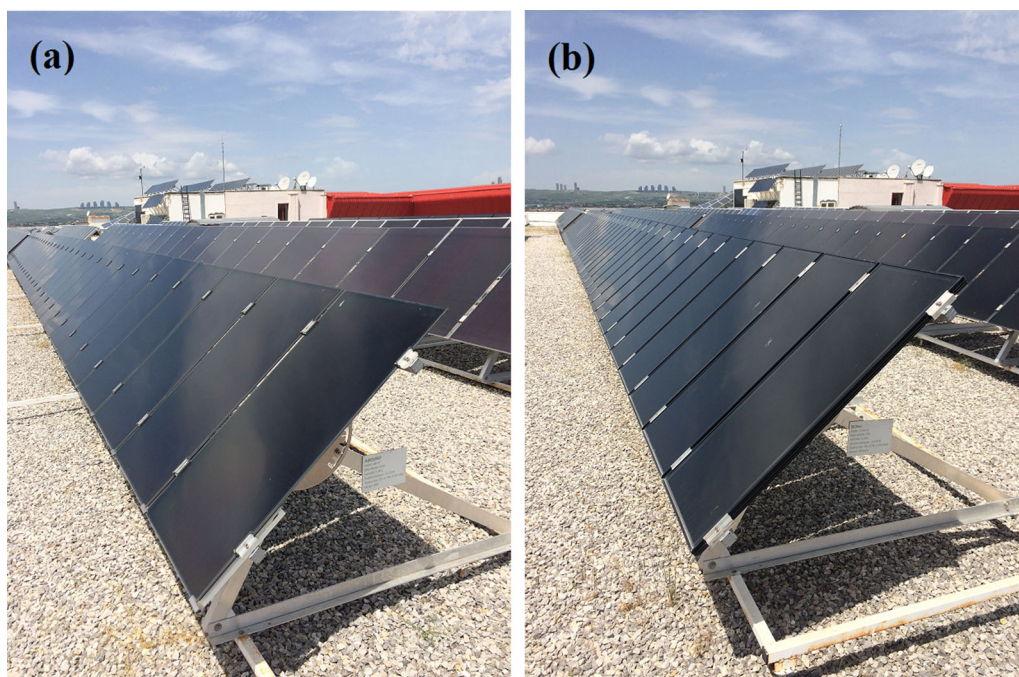
Fig. 2. Experimental setup at Gazi University Golbasi campus Technopark: (a) CdTe thin-film module string and (b) CIS thin-film module string.
