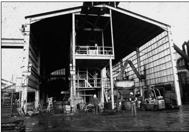
Fig. 8—Commercial tin slag reduction plant at ATS.
