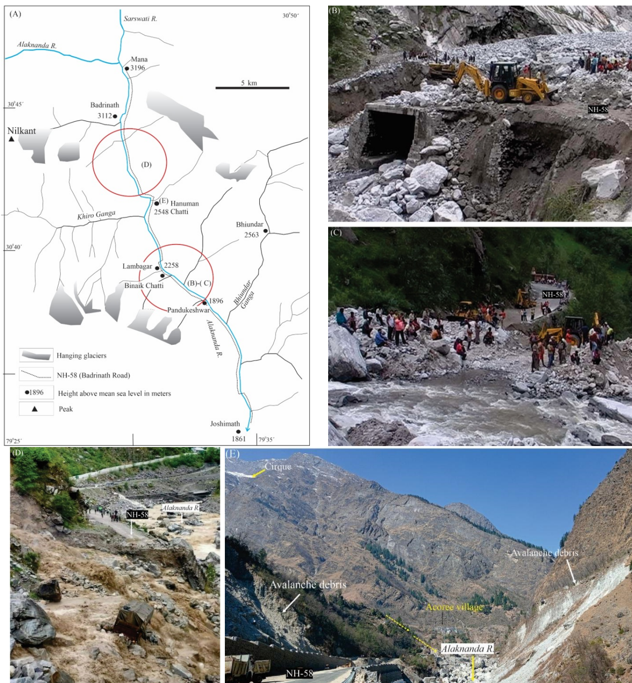
Fig. 6 (A) Geomorphological map of sector-3 between Binayak Chatti and Lambagar showing many hanging glaciers. Glacial erosion generates (para)glacial sediments in the valleys which frequently damage the road. For example, (B) and (C) show the damaged NH-58 near Binayak Chatti after the summer rainfall of 2009. (D) On 21st May 2021 NH-58 was completely washed away near Lambagar by paraglacial sediments transported by a glacial-fed stream Khiro Ganga (E) A new buttress wall near Binayak Chatti was built recently to protect the road which was frequently damaged by the mobilization of unconsolidated para glacial sediment particularly during monsoon season. Height above mean sea level and village name (black dot) and peak (black triangle) are also marked.
