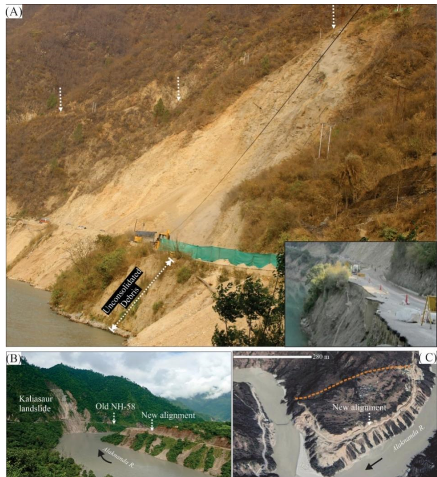
Fig. 4 (A) Photograph of Pharsu landslide developed on highly sheared quartzite on NH-58. The white arrows indicate the new road alignment proposed before the commissioning of the road which was not completed. The subsidence and lateral erosion of NH-58 caused due to the Reservoir Drawdown effect near the Srinagar hydropower dam (shown in the inset). (B) The chronic landslide of Kaliyasaur could not be treated despite several engineering measures over the years and had to be bypassed. (C) Google imagery of the newly aligned NH-58 built on unconsolidated fluvial terrace gravels indicates the new road's susceptibility to subsidence and toe erosion. Field investigations indicate that the road alignment above the village over solid bedrock (orange dashed line) would have been safer.
