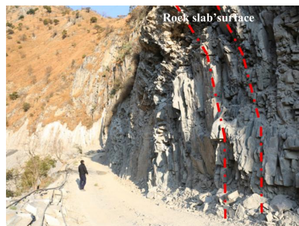
Fig. 2 Toppled rock mass of the highway slope at Miaowei hydropower station.
