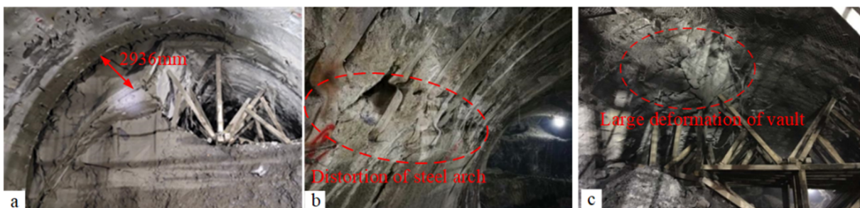
Fig. 4 Failure characteristics of rock surrounding of No.2 inclined shaft.
