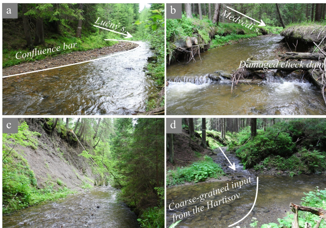
Fig. 2 (a) – Confluence bar associated with the Lučný stream (LU), (b) – damaged check dam immediately downstream of the confluence with the Medvědí stream (ME), (c) – one of several bank failures in the upper part of the study stream reach based in claystone lithology, (d) – confluence with the Hartisov stream (HA).
