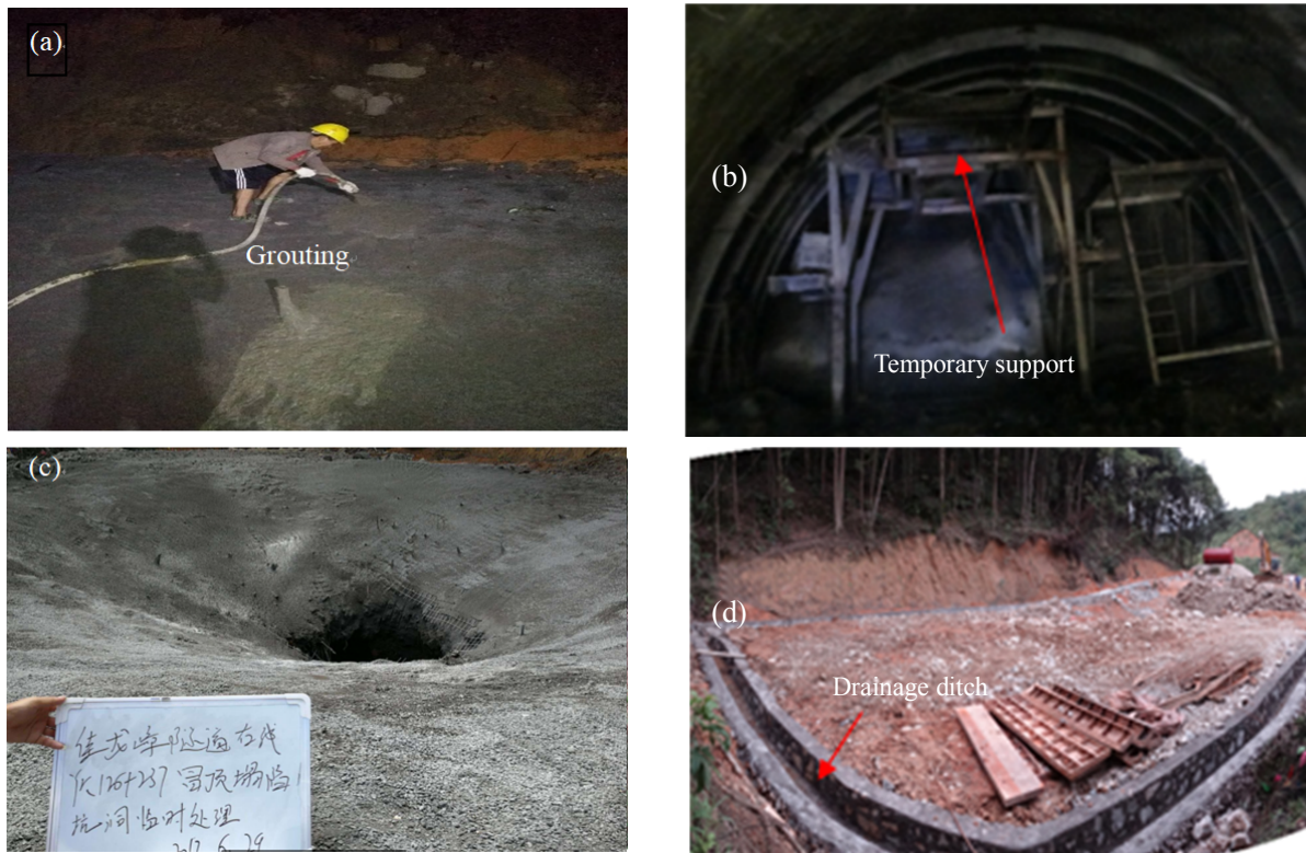
Figure 12 In situ photographs showing implementation of the countermeasures. (a) Grouting reinforcement; (b) Temporary support; (c) The surface is covered with reinforcement mesh; (d) Round drainage ditch.
