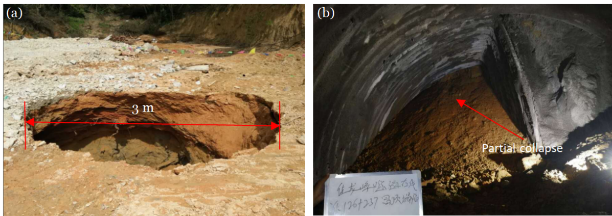
Figure 4 Collapse field of section YK126+237; (a) Tunnel roof fall. (b) Collapse of tunnel crown.
