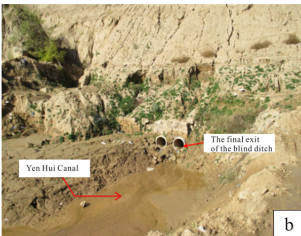
Figure 4 The blind drainage system in Yan'an New City: (a) layout of the blind drainage system; (b) the final exit of blind drainage.
