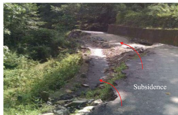
Figure 7 Subsidence near Pyarieni Jhora (Tilt Sensor 2) and ground (Dikshit et al. 2018).
