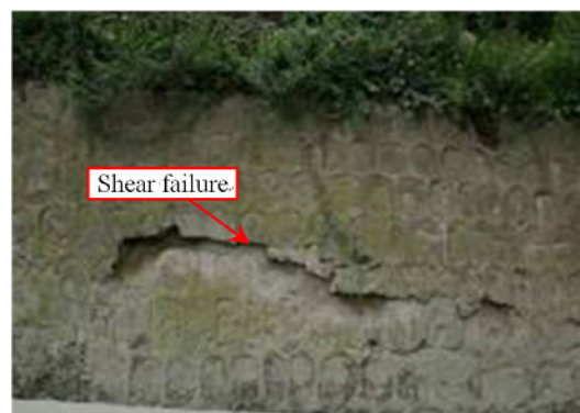
Figure 7 Shear failure of a stone retaining wall.
