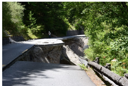
(b) The subgrade damage
