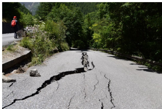
(a) Road-surface damage
