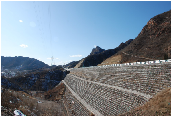
Figure 1 Photo of a geosynthetic-reinforced slope (in Beijing-Chengde highway, taken by Tensar Geosynthetics Limited Company in 2009).
