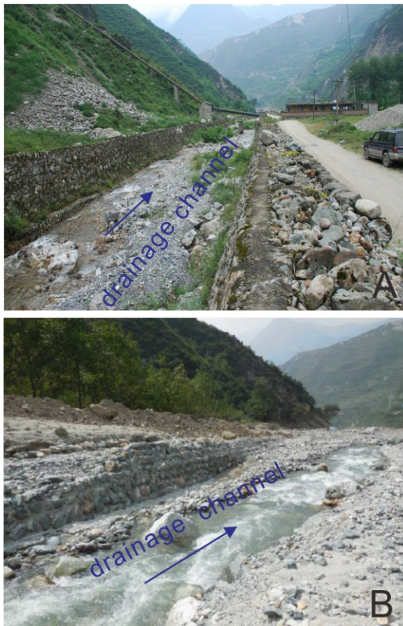
Figure 11 The drainage channel before and after the debris flow event.
