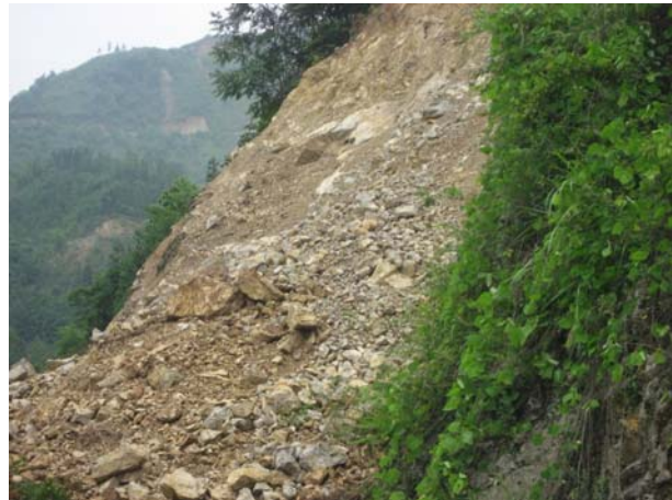
Figure 5 Surficial failure of rock slope
