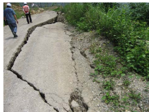
Figure 7 Development of cracks along the road indicates the instability of down slope of the road
