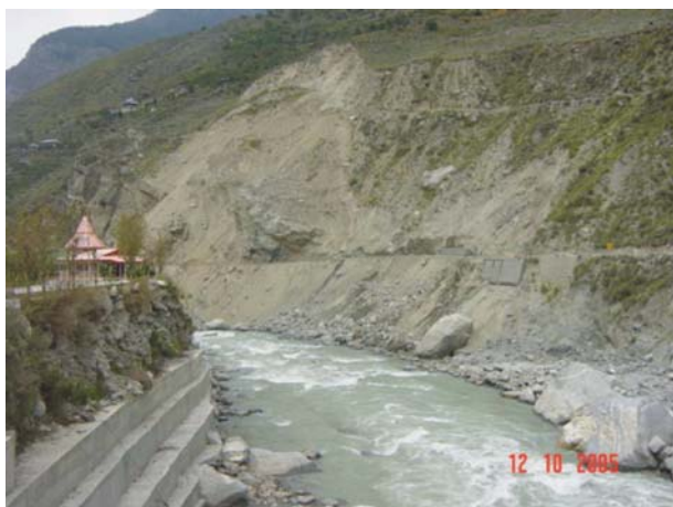
Figure 6 Translational debris landslide located about 200 m upstream of the Tapri Village affecting the NH-22 and the link road to the Tapri Village.
