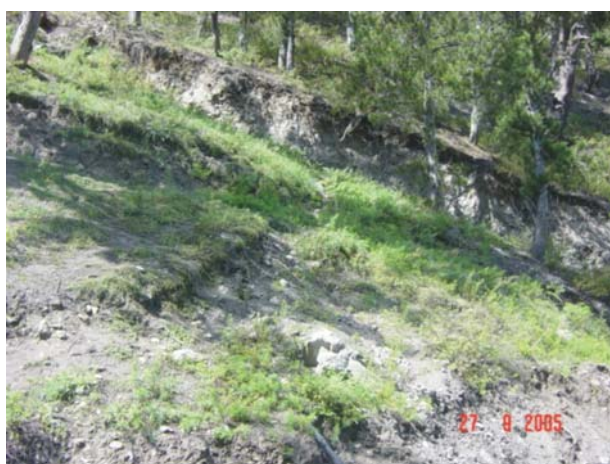
Figure 9 Scarp of the Telangi Farm House Landslide which is about 3 m high.
