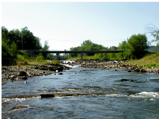
Fig. 12 View of the uppermost part of the study reach where recent, deep channel incision has induced backward erosion threatening the bridge
