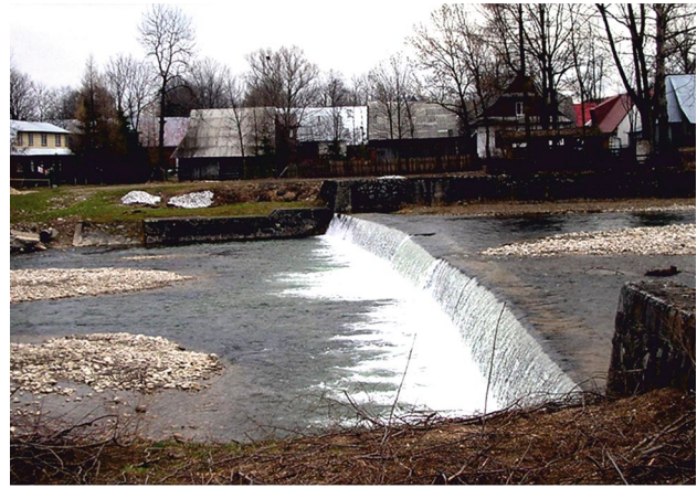
Fig. 11 High weir constructed at the downstream end of the study reach in the early 1960s that has induced bed aggradation in the lower part of the reach
