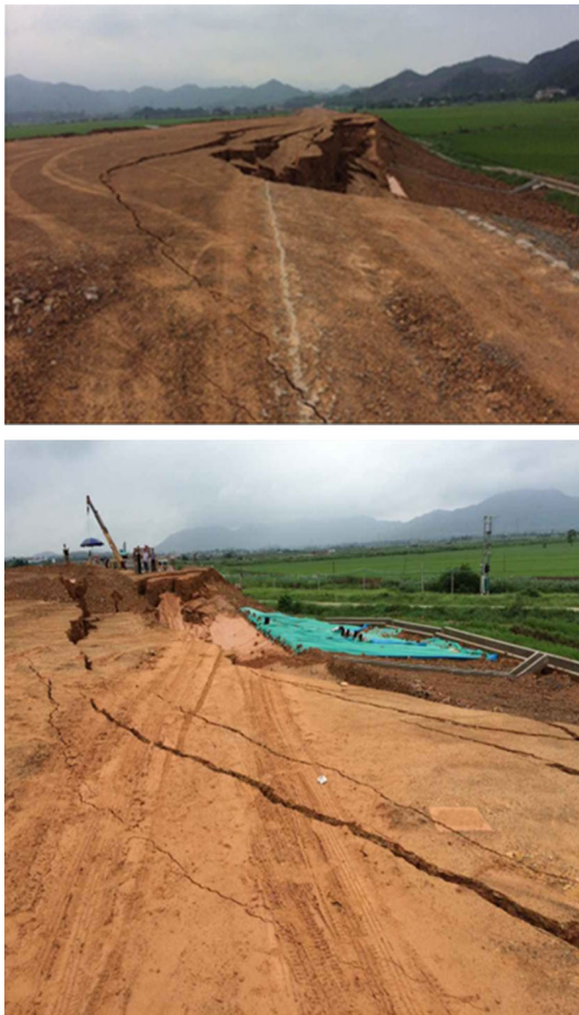
Fig. 1 Photographs of instability failure of rigid pile composite foundation under embankment
