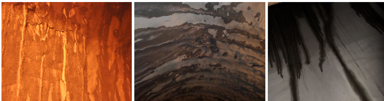
Fig. 3 Failure characteristics of Lanjiayan tunnel
