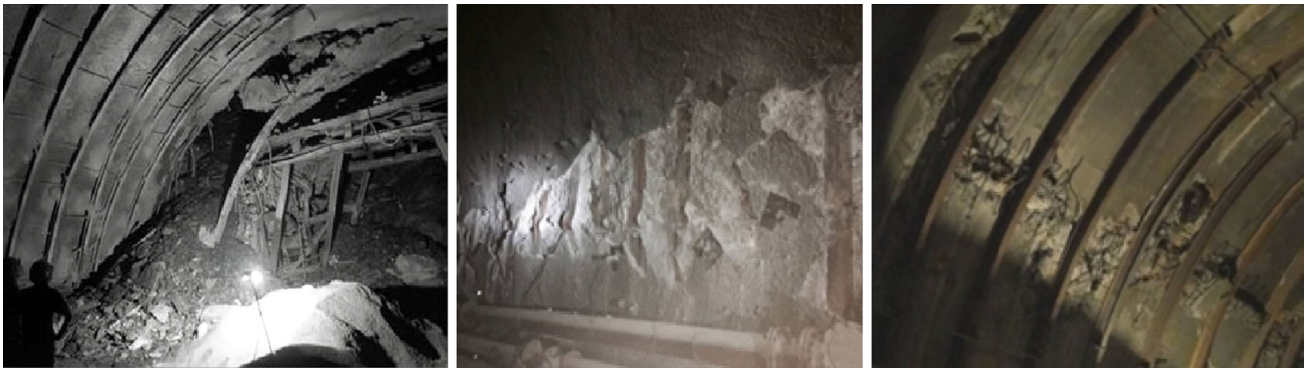
Fig. 1 Deformation and failure characteristics of typical deep-buried carbonaceous slate tunnel
